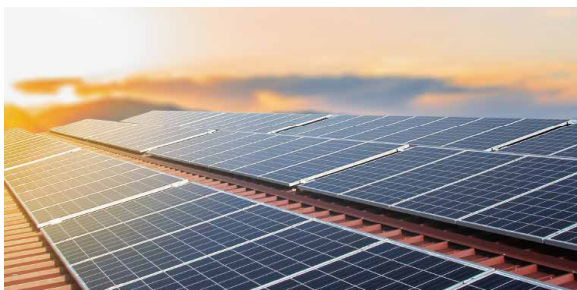
Installation of Solar Panels on Roofs for Energy Saving and Consumption Reduction
